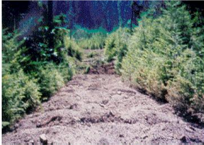
Example of hummocky surface on a road immediately after scarification by an excavator bucket. Photo from MARD Road Decomm Monitoring Report.
