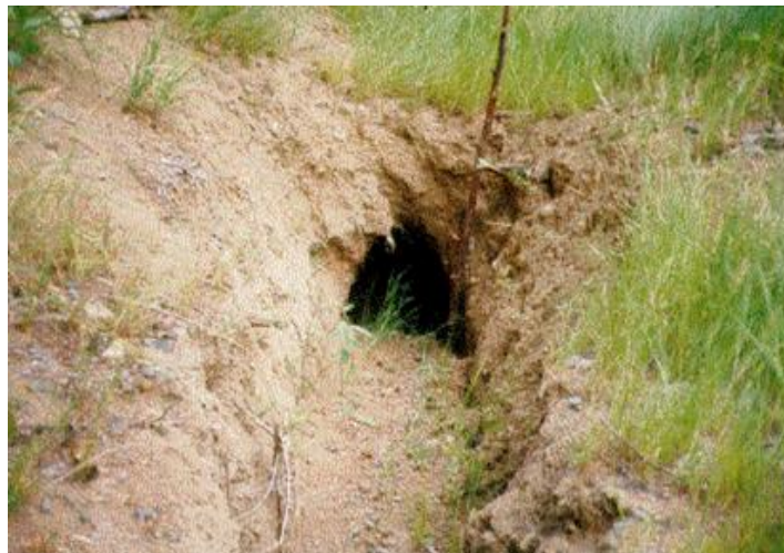
Example of culvert section and associated fill that was not fully removed. Photo from MARD Road Decomm Monitoring Report.
