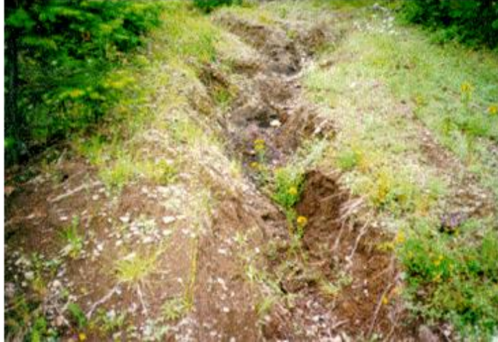
Example of erosion (deep gully). Photo from MARD Road Decomm Monitoring Report.
